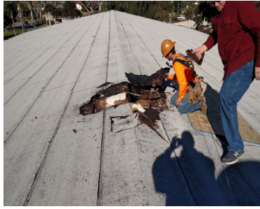
Rotted Wood Roof Framing
